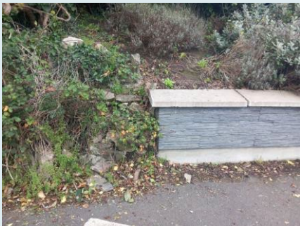
Top and above: The use of thick cement pointing and thin veneer and tile cladding presents a very different character to traditionally constructed limestone walls.
